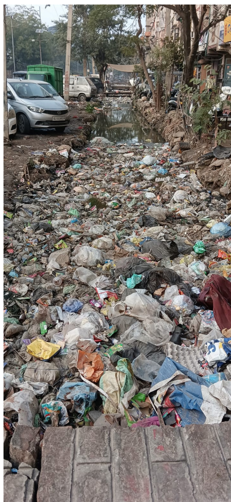
Photo 5 - Open Drain, Abul Fazal Enclave.
