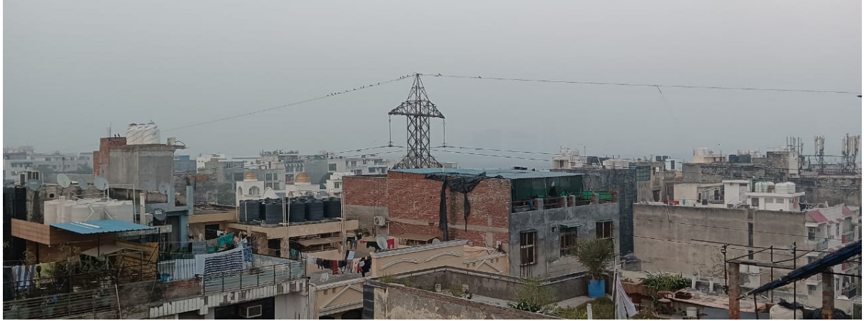
Photo 7 - High Tension Wire, Hari Kothi
